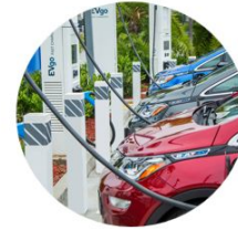
Electric Vehicle Charging
